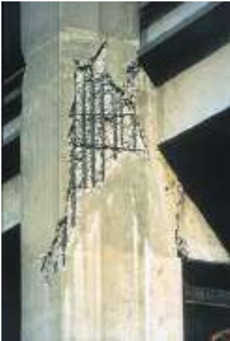
Lap splices transfer their load through the concrete and will fail as concrete cover degrades.
